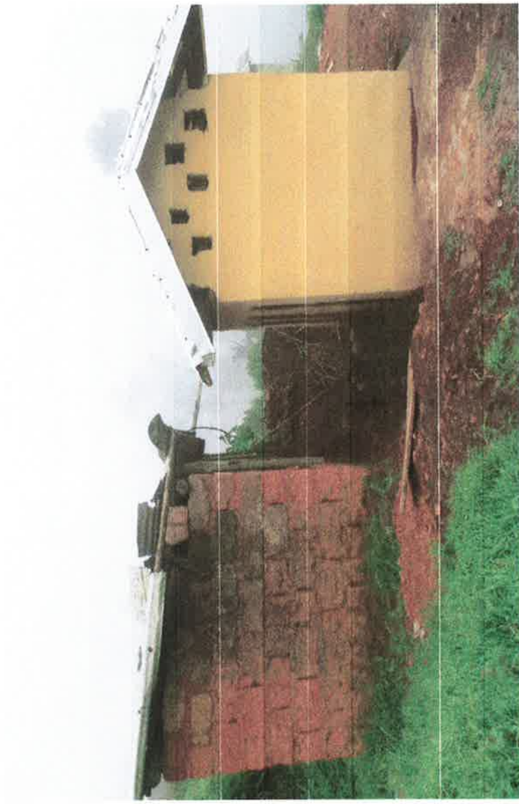
Government Primary School Marita: Latrine situation before and after CIC & ICA intervention
